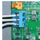
Figure 1. Remote Pool-Off-Spa Connection (3-Wire Connection)
